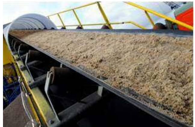
Misaligned drums and idlers cause extra wear / 調整不備のローラーやブーリは過剰摩耗の原因
