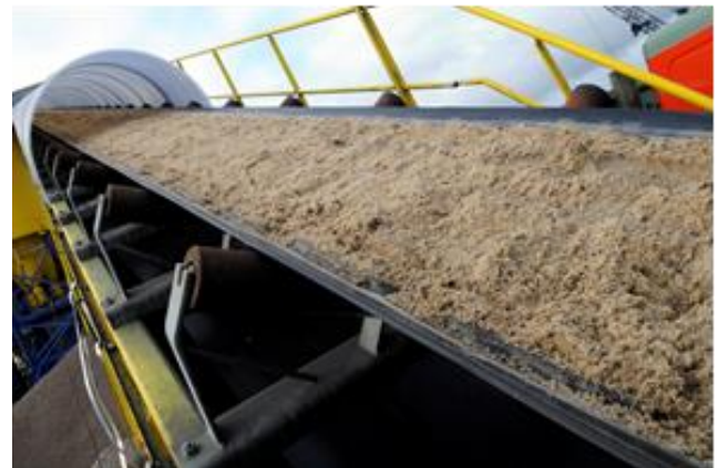
Misaligned drums and idlers cause extra wear
