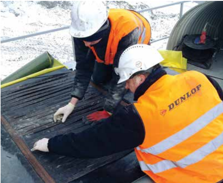
Those physically working with conveyor belts need to be safeguarded.
